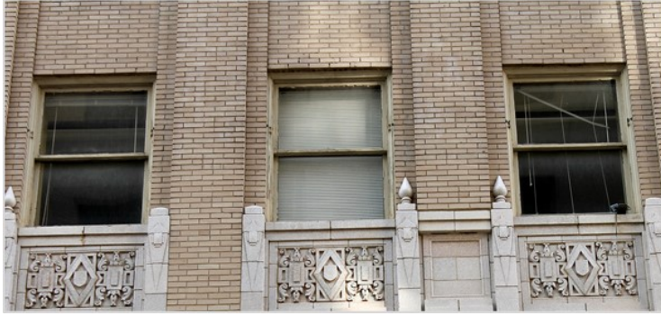
1. Wood Double-Hung Windows
